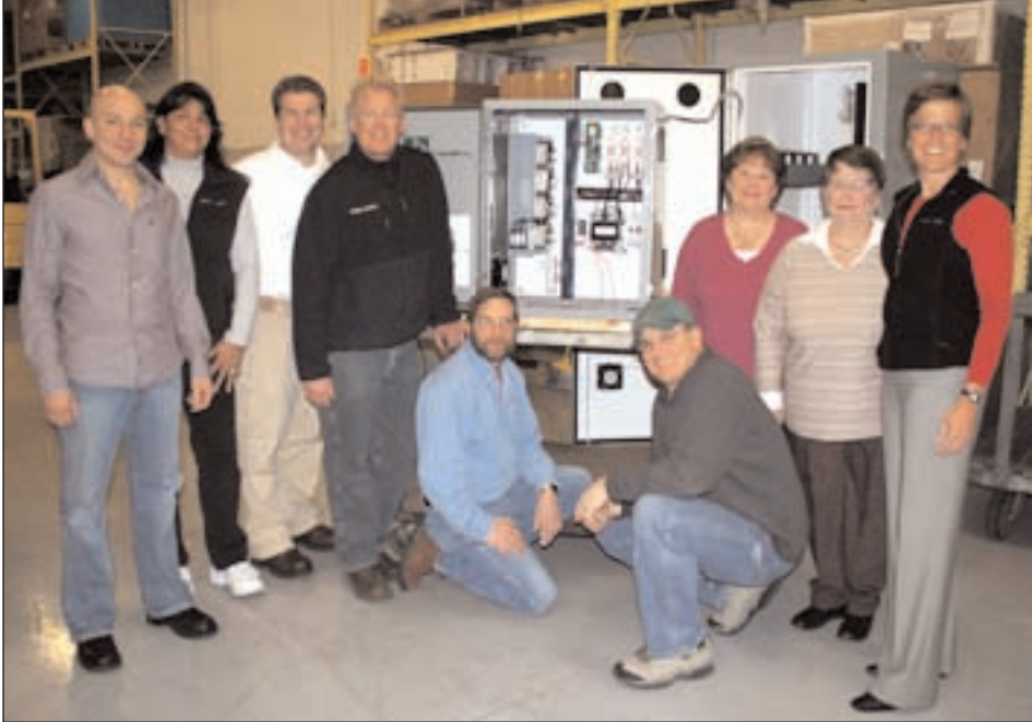
Myron Zucker, Inc. in Sterling Heights provides power solutions to a multitude of customers.
